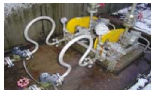
Bent type kerosene piping
