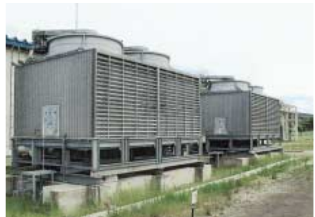
Operation of one of the two cooling tower units could be stopped thanks to the improved operation efficiency achieved
