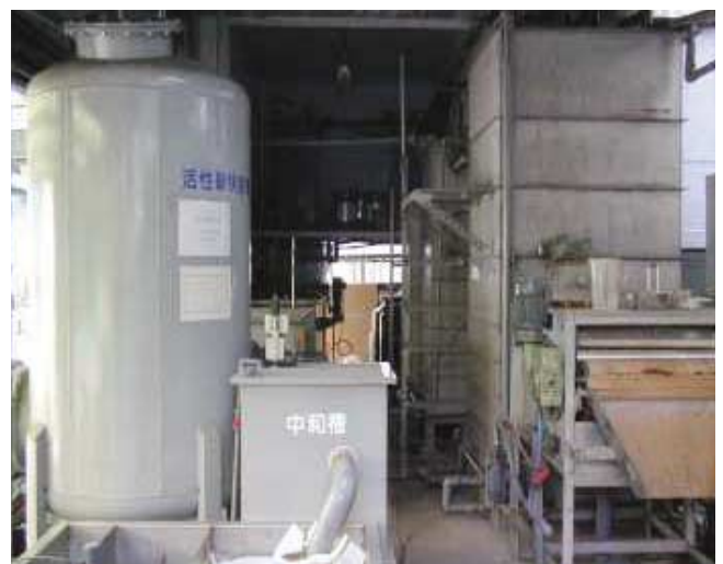
Newly installed wastewater processing facilities
