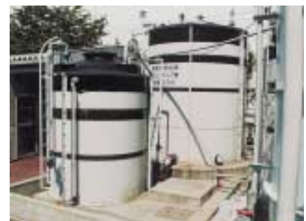
Temporary recovery tank
