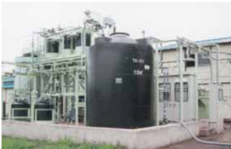
Wastewater processing unit
