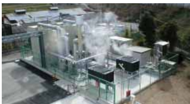
Private generation facilities
