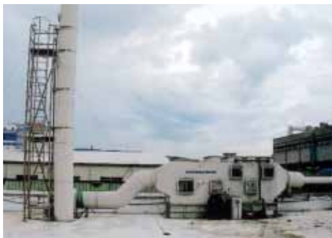
Organic solvent waste processing facilities.
