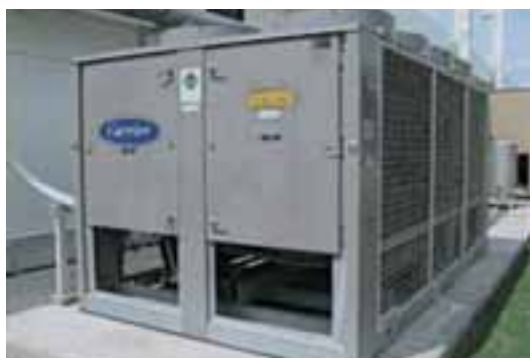
Non-CFC type new chiller unit
