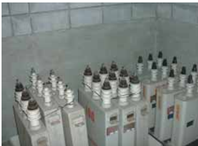
Storage for equipment using PCB
