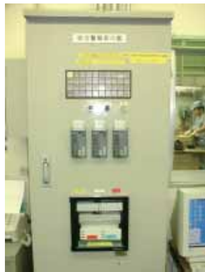
Integrated monitoring cabinet for the environmental facilities, etc. (Sendai Plant)
